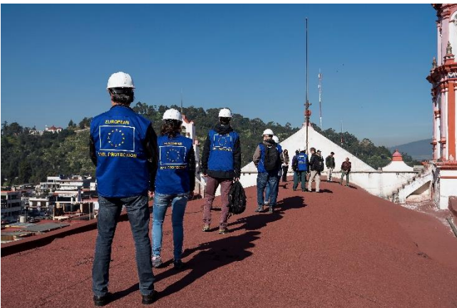
EUCP Team experts during the damages assessment on the Parish of the Asunción following the earthquakes of September 2017 © Miquel San Nicolás
